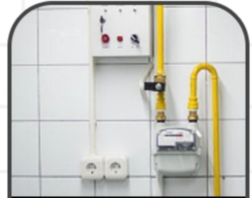
Gas Meter & Solenoid Valve
