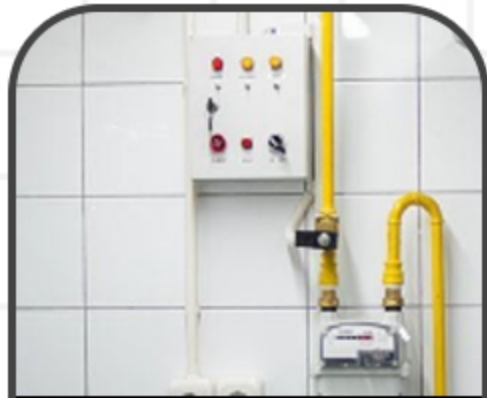
Safety Gas Alarm
