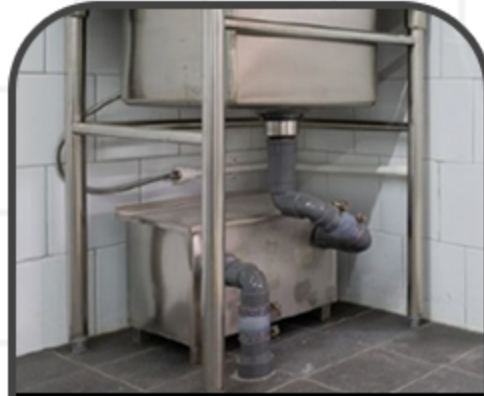
Grease Trap (Dibawah Sink)
