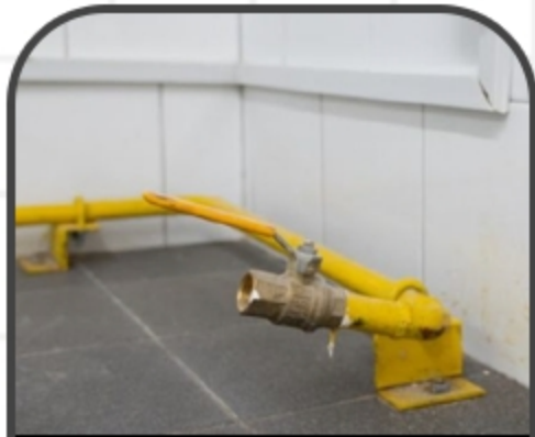
Gas Valve & Detector
